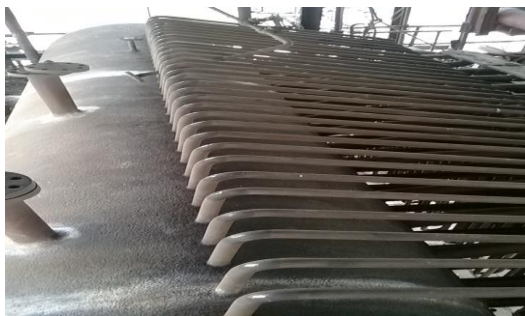
Fig.1 Actual photograph of Steam drums of a super heater
