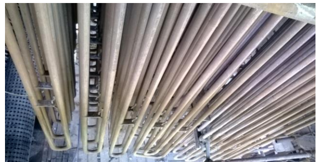
Fig.2 Actual photograph Super heater tubes of a boiler
