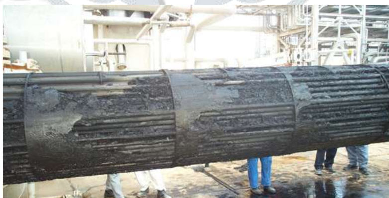
Figure: Fouling of Heat exchanger
