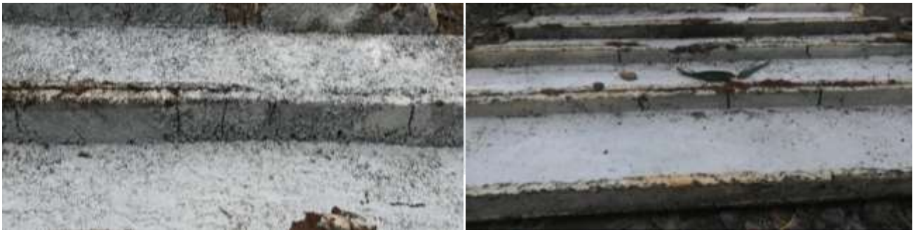
Fig.14Crack pattern on Web of Closed Channel Slab S_2 Fig.15Crack pattern on Web of Closed Channel Slab S_3 .
