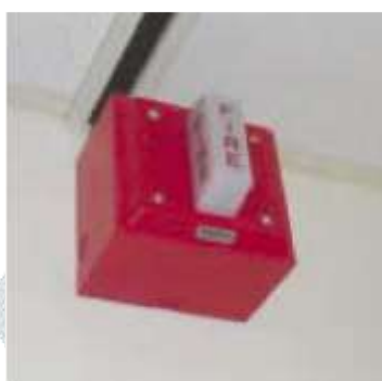
FIGURE - 1.2: Control Panel. (Source: OSHA: 3256 – 07N - 2006)
