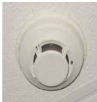
FIGURE - 1.1: Initiating device (Smoke detector)
