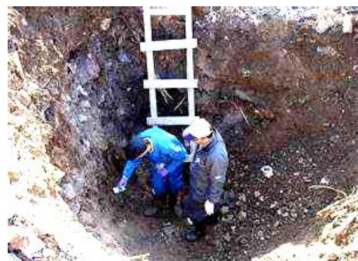
Figure 5. Shows the excavation processes in Khan Neshin area. This process fulfilled for purpose of determining the concentration of uranium in mother rocks. Source: Xinhua News Agency.
