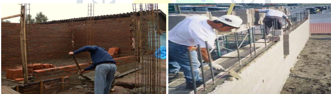
Fig. No. 4 Masonry building technologies: Confined masonry construction in Chile (S. Brzev, left), and Reinforced masonry construction in Canada (B. McEwen, Right) (Ref. Meli R. et. al 3 )
