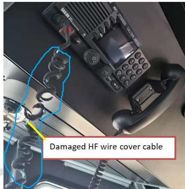
Figure 4 damaged wire cable of HF.
