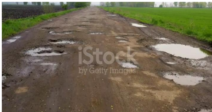
Fig 3: Before detection of potholes
