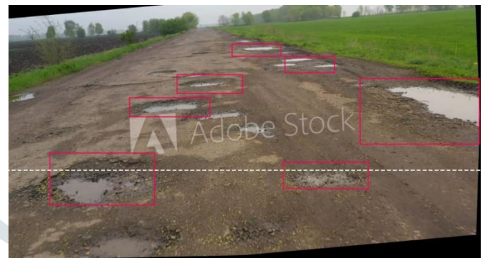
Fig 4: After detection of potholes
