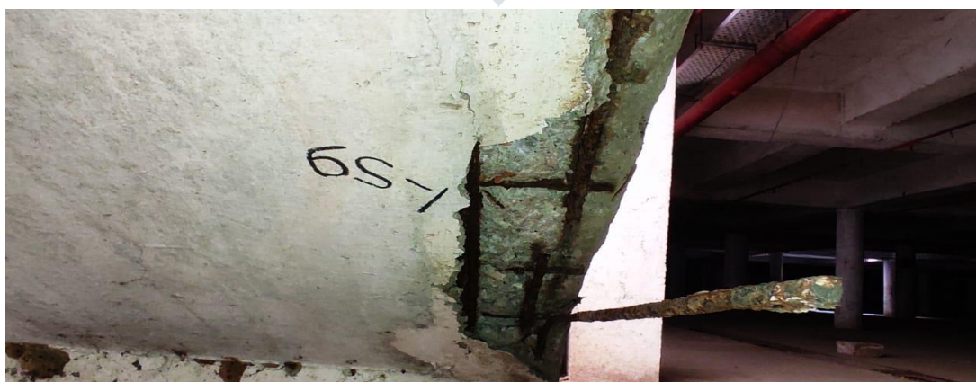
Fig-8 Staircase with exposed reinforcement
