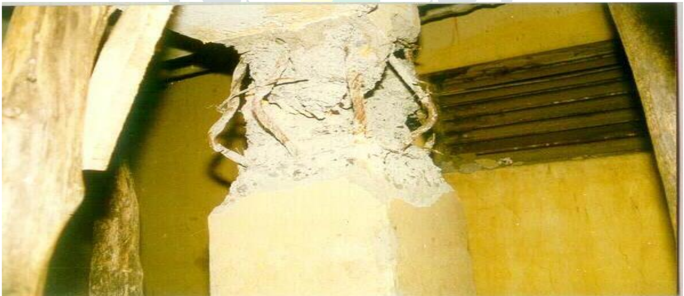
Fig shows Damage to Column
