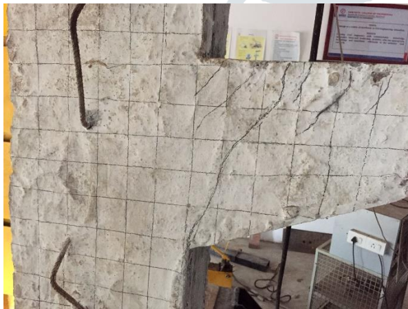
Fig .7: Crack on Control Specimen
