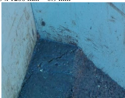
Fig. 6: Initial failure in slope at 50 minutes
