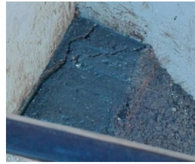
Fig. 7: Progress in failure on PWP increase at 133mm/h rainfall intensity
