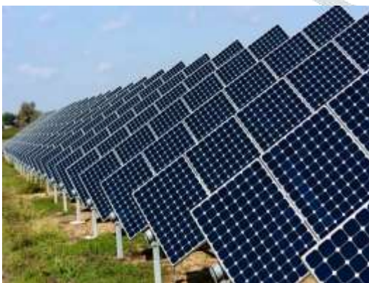
Fig. 3 Photograph of solar array installed
