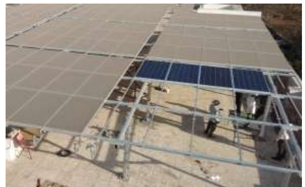
(Fig 09, array mounting structure, ref- sakal office plant)
