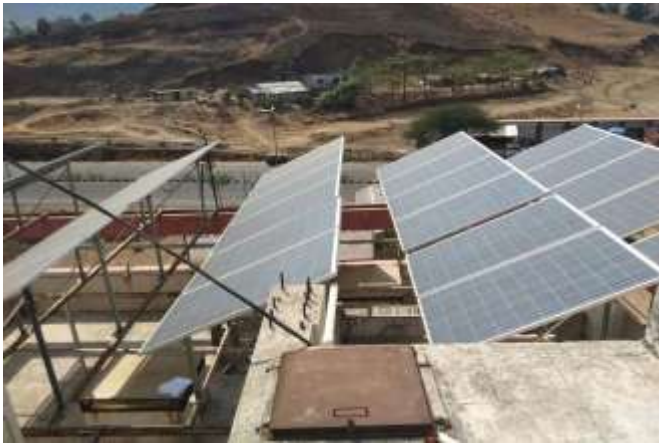
(Fig 12, roof top plant visit, ref-hotel warunse)
