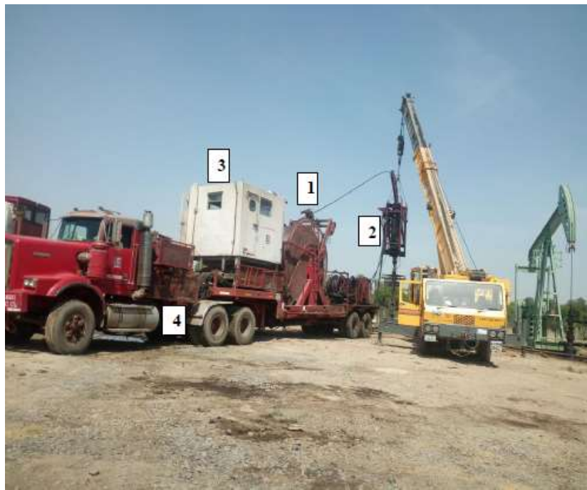
Figure 3: CT Unit in operation.
