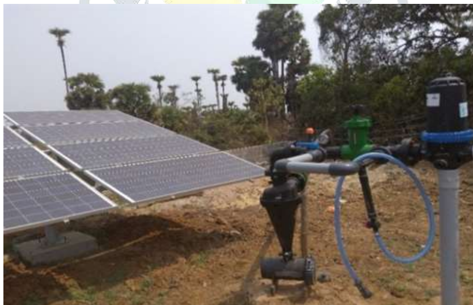
Fig.13. solar water pumping system at vizianagaram district
