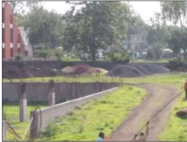
Fig 3.4: Excess storage of Sand and Aggregate
