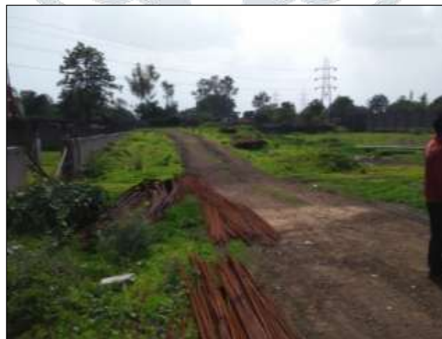
Fig 3.3: Excess storage of Steel
