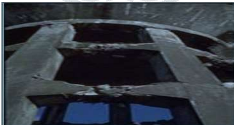
Fig. 1.1: Bending Shear Failure in beam
