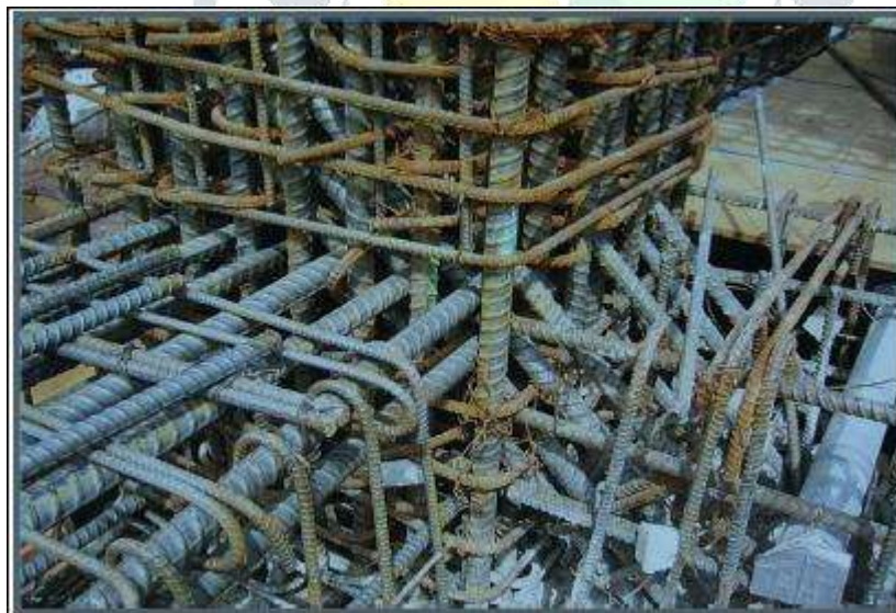
Figure 1.15 Congestion at the Beam-Column Joints (ref.: www.concreteconstruction.net )
