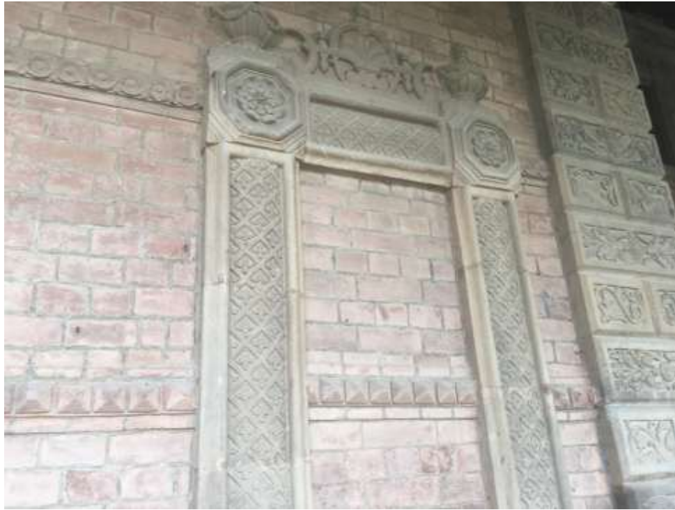
Plate 7: The picture of a wall of the Heritage Hotel which is designed with artistic architecture and different types of designs.
