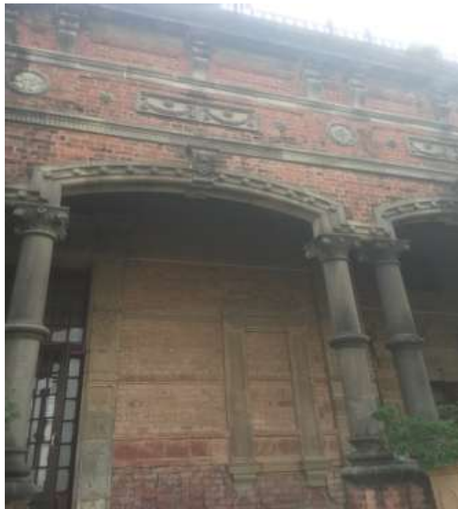
Plate 10: The image of a outer Barandah of the Heritage Hotel with proper designs.
