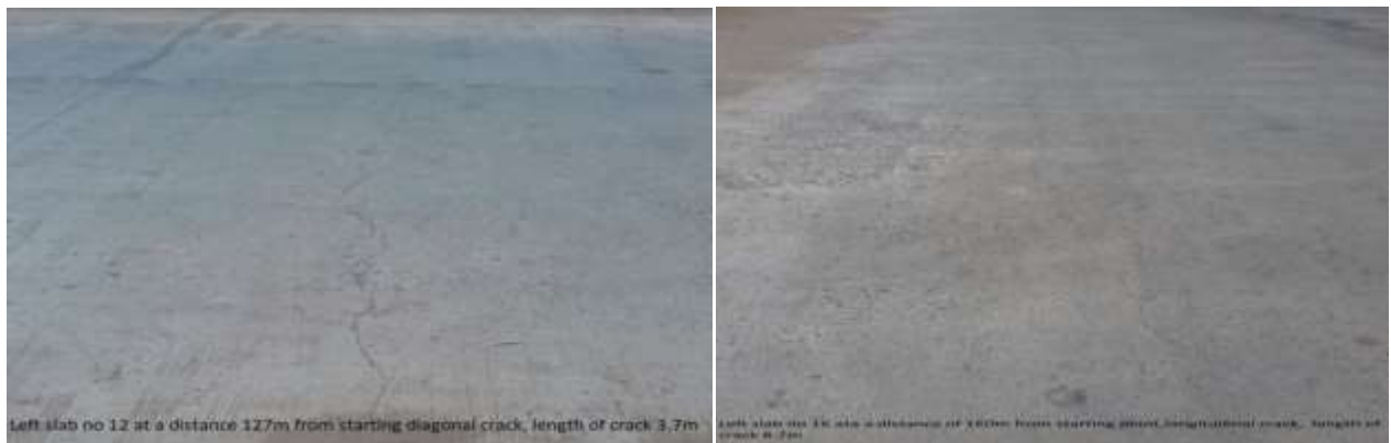
FIG: 1.4 – LOW SEVERITY L/T/D AT TWO ROAD SLABS.
