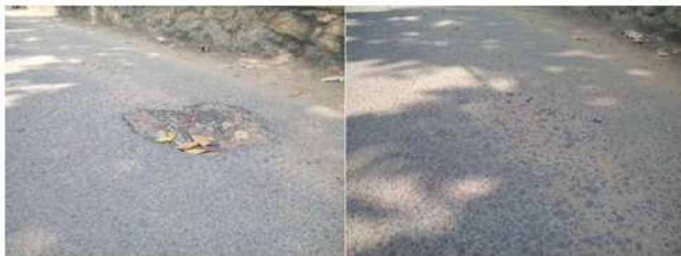
Fig. 12 Potholes and raveling on control road section
