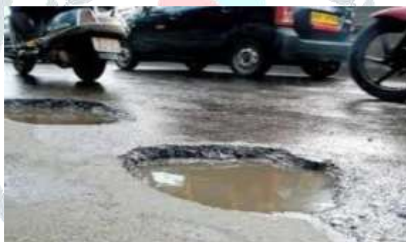
Fig 1. Condition of Indian roads with potholes.
