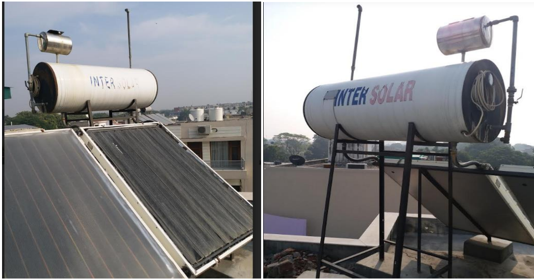
Fig 2. Front and rear view of a solar geyser unit fitted atop a roof of a house in SAS Nagar Mohali (Punjab) subsidized by PEDDA, functional since December 2016.
