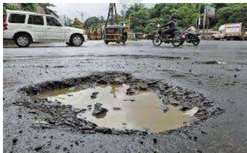
Fig 1. Indian roads with potholes.
