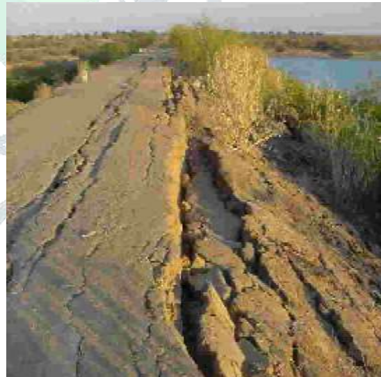
fig 2: failure of upstream crest of fategadh niigata, dam, (courtesy of iit kanpur)[1]
