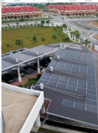
Monocrystalline PV modules (27kWp) on the carpark roof
