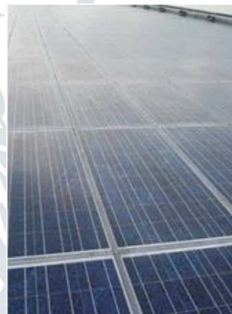
Polycrystalline modules (47.28kWp) on the main roof
