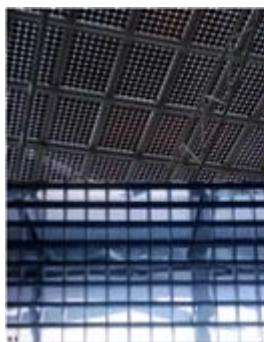
Glass semi-transparent PV modules (11.64kWp)
