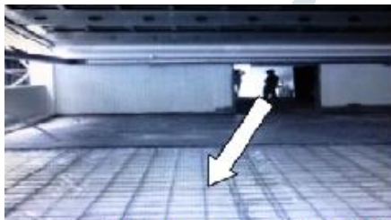
Polystyrene layer is installed on the uppermost floor of the office building (Source: Malaysia Green Technology Corporation, 2010)
