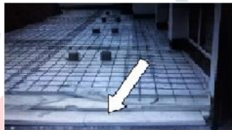
The photo showed the installation of Styrofoam during the construction of the roof.
