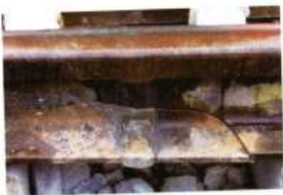
Fig. 1 - Horizontal Flaw in Web through Weld
