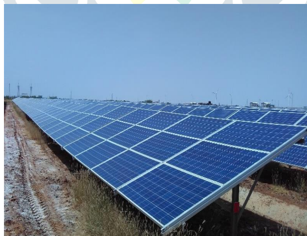
Fig 3: Multi-Crystalline PV Panels
