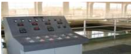
water treatment filter control panel
