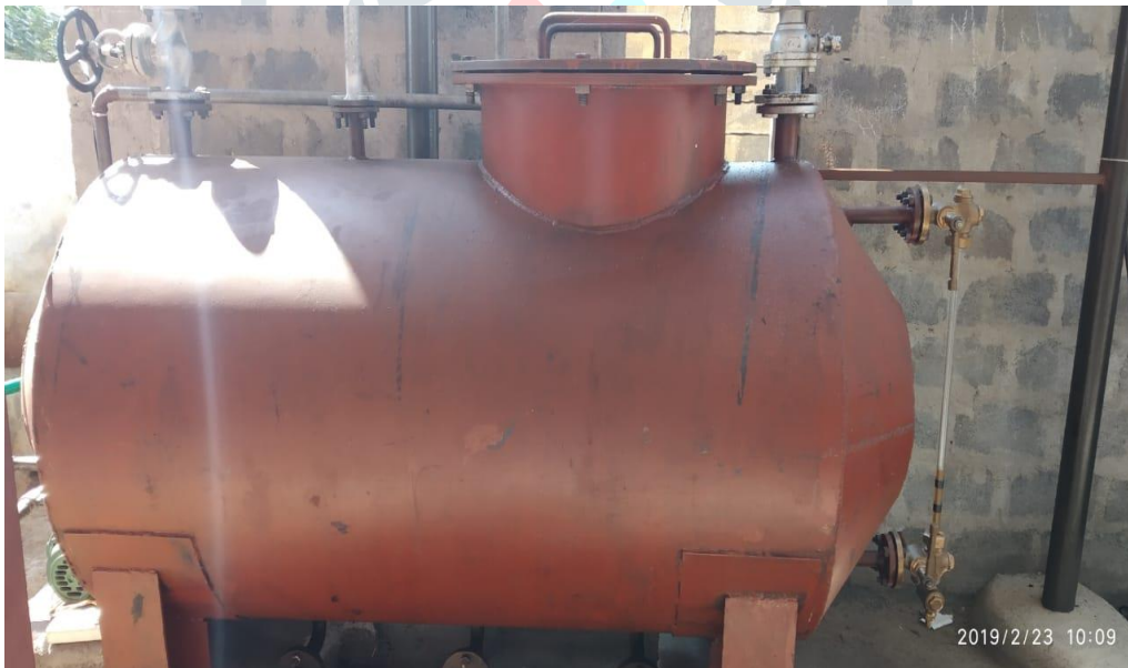
Thermic fluid tank
