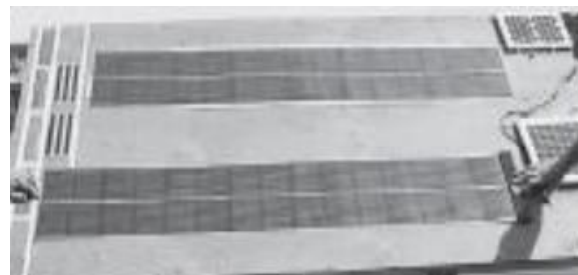
Figure 5: Infrared plastic solar cell on the rooftop
