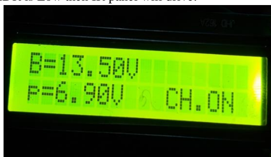
Fig5., Charging Of battery display on LCD
