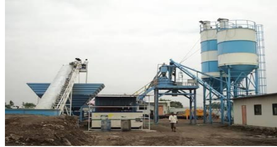
Fig 2. Manual Batching Plant
