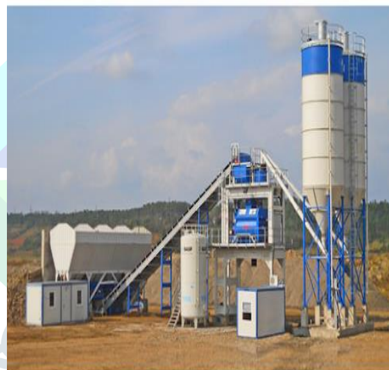
Fig. 3. Semi- Automatic Batching Plant
