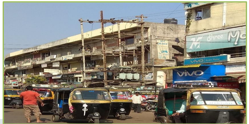
figure 9 Open Wire Electricity supply
