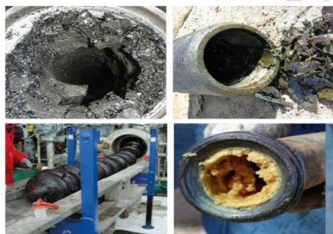
Fig.1 – Blockage in Crude Oil Pipelines
