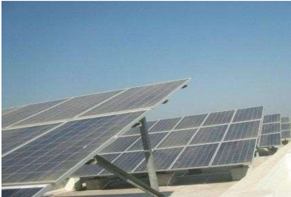
Figure 5 25KW Solar PV power plants at SewaBhawan, R.K.Puram, and New Delhi
