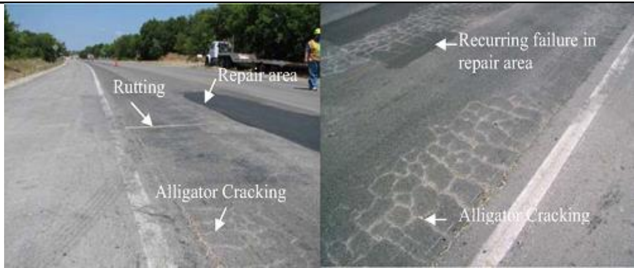
Figure: 1 Pavement failure (Source-Google)
