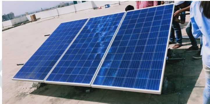
Fig.3: Solar charging station
