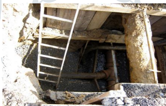
Fold in sewer connection
