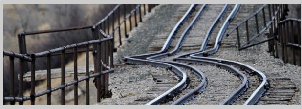
Fig 1. Shows the buckling of rail tracks
