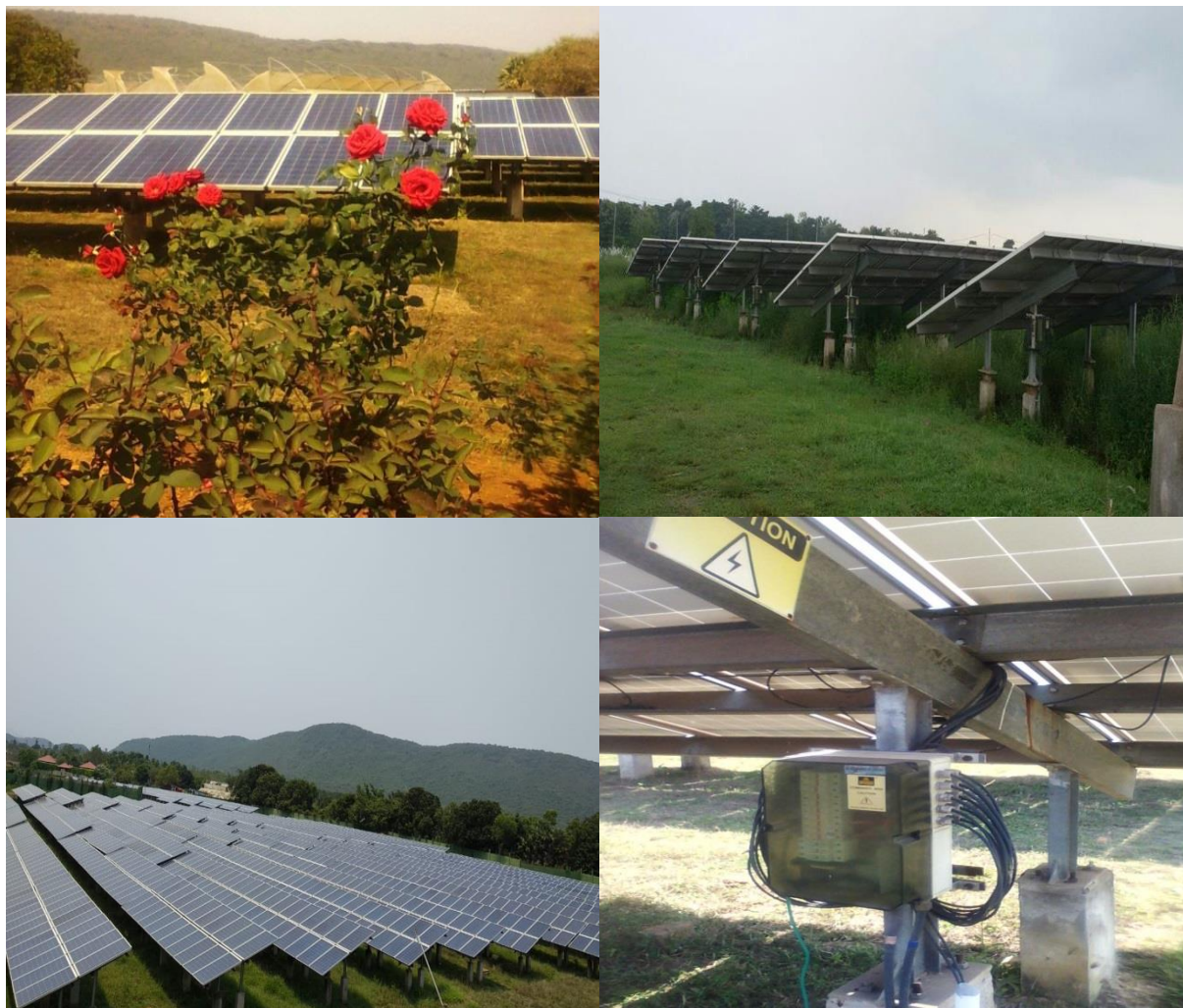
Figure 4.1 1 MW Gross metering Solar power plant, Khurda and Cuttack, Odisha
