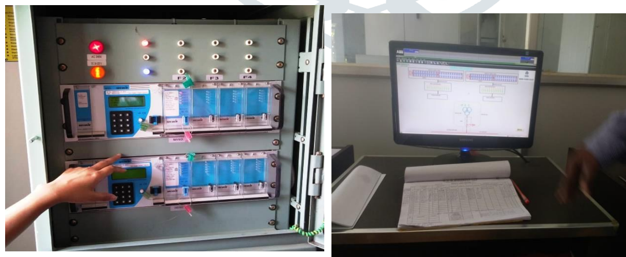
Figure 4.2 1 MW Gross metering Solar Power Plant Control room, Khurda, Odisha
