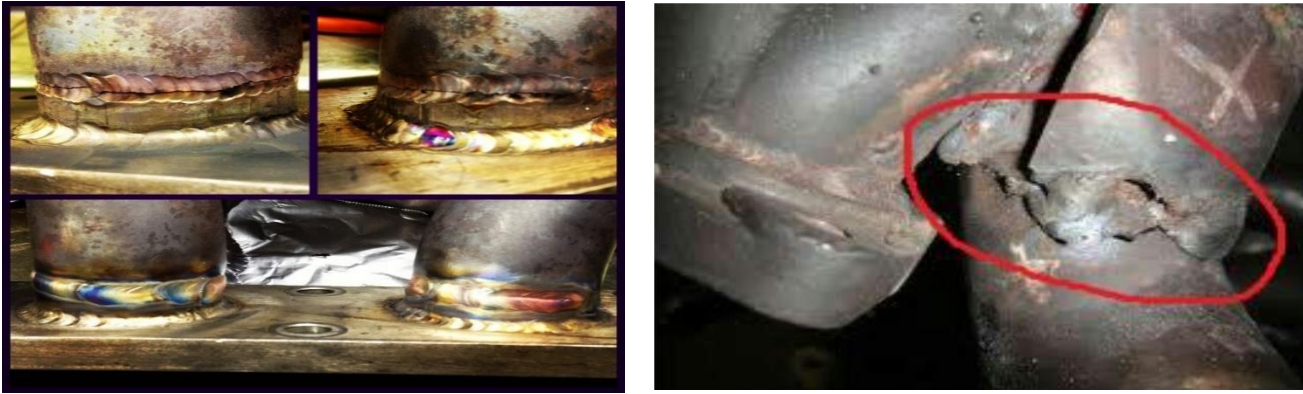
Figure 01, 02: cracks in connections due to thermal stress
