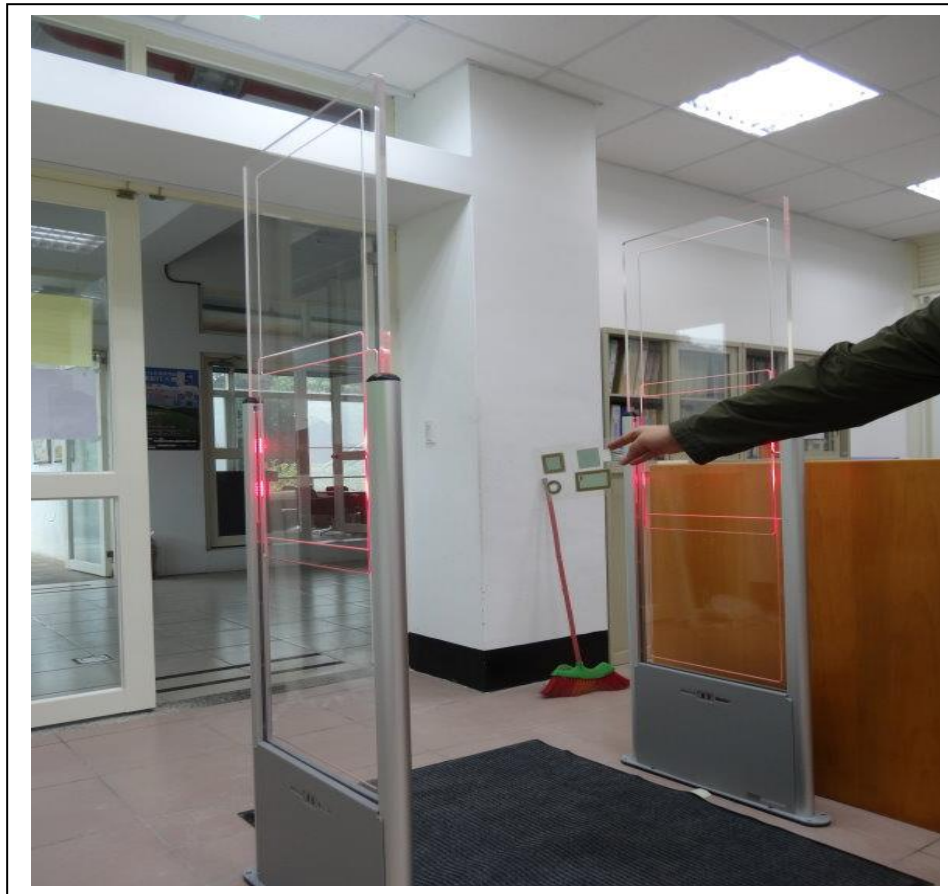
Library RFID System - UHF Detection Gates
