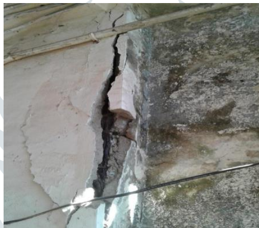
Fig 2: Cracks in structural members due to corrosion
