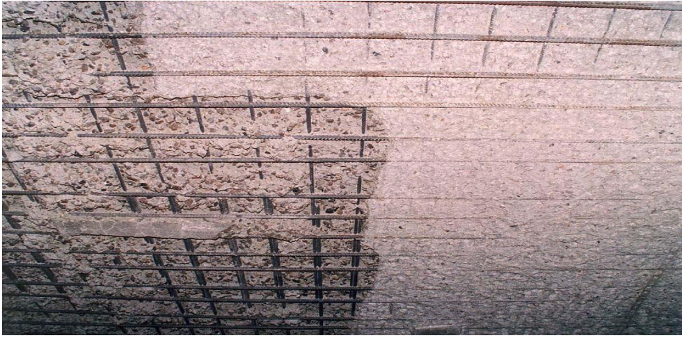
Fig.1 Fire Damaged Slab
