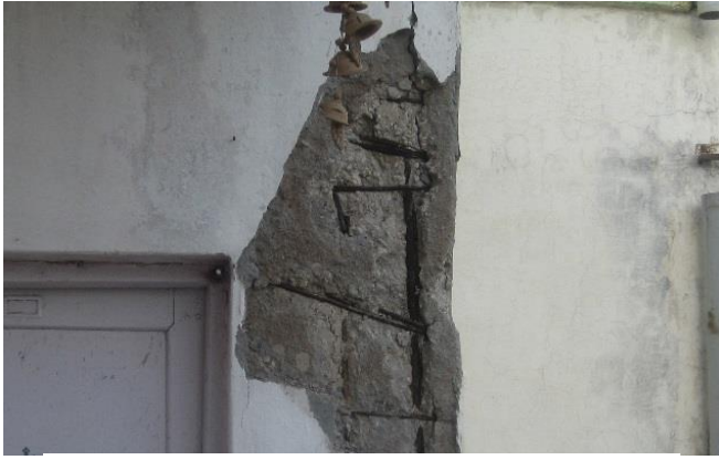
Figure 3 Corrosion in steel
