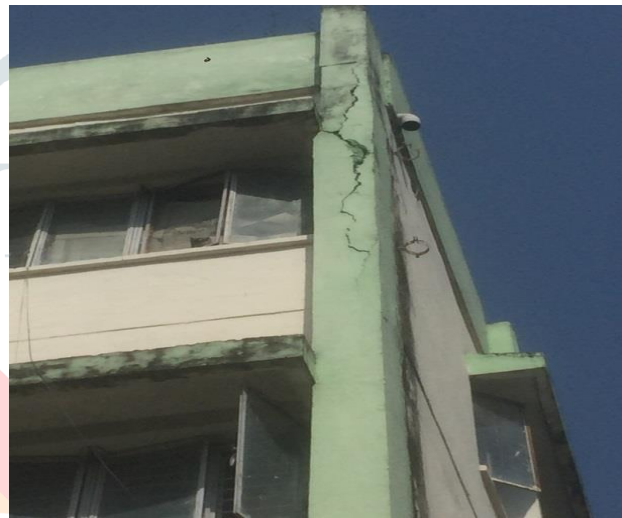
Figure 6 Vertical crack on column
