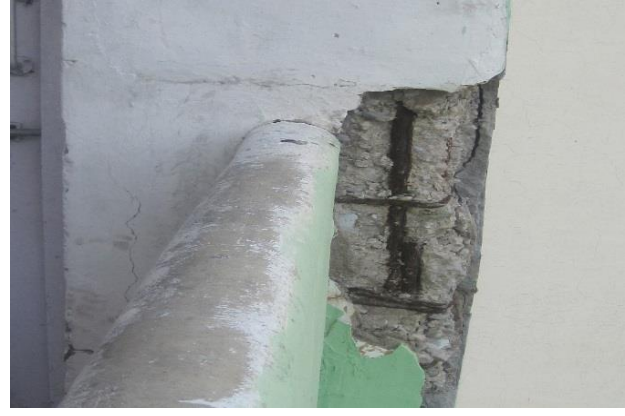
Figure 4 Spalling of Concrete
