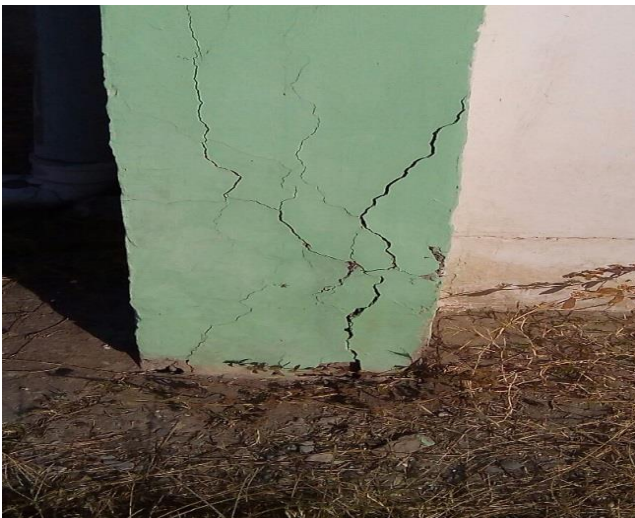
Figure 5 Hair Line cracks in column
