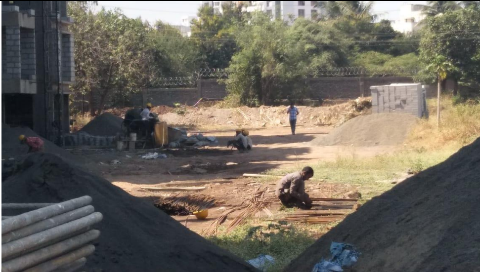
Figure 4.2 Worker doing work without safety Helmet
