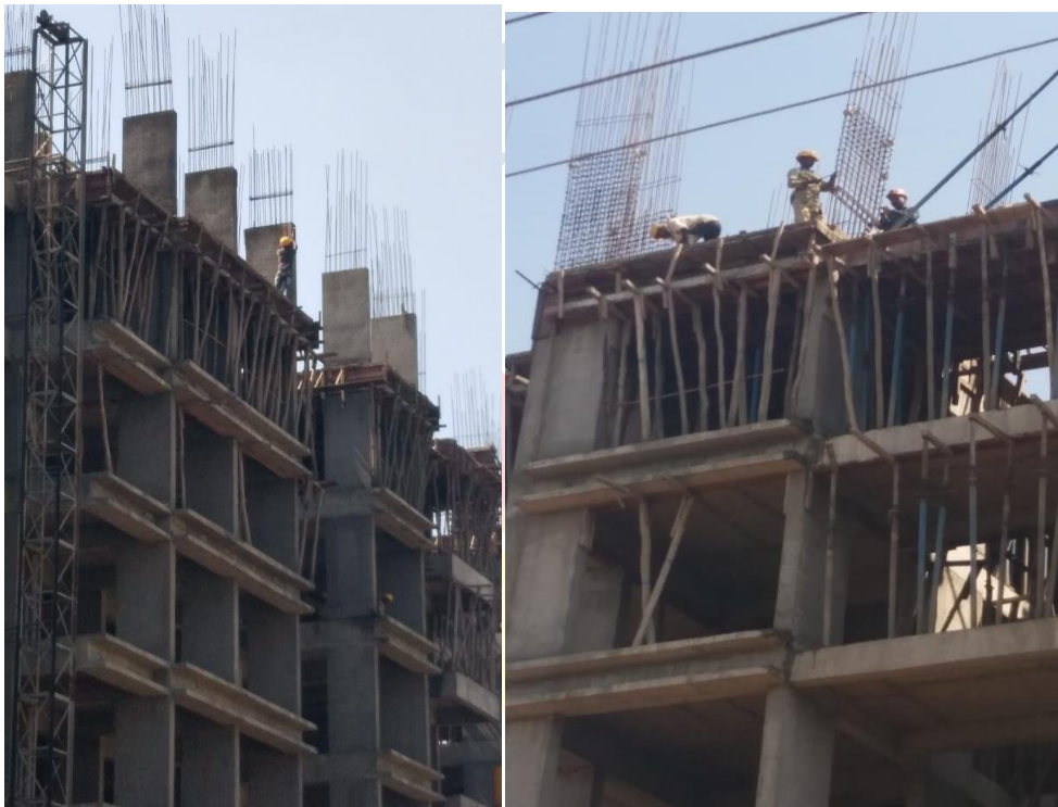
Figure 4.3 Workers work without safety belt, gloves and any precaution
