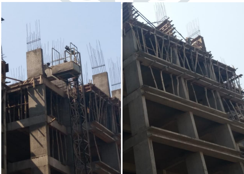
Figure4.1Workers doing work without safety belt
