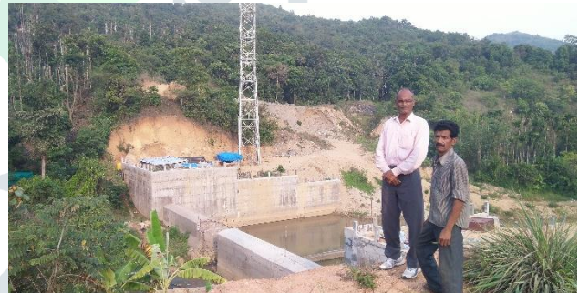
h) View from U/S of weir under construction near Aluvalli across Yettinahole at D/S.
