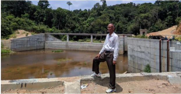
e) U/S of weir constructed inside the Kadumane estate across Kadumane estate Halla - 2
