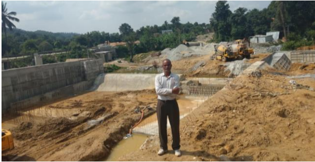
c) D/S of weir under construction at Maranahalli village across Heggadde Halla
