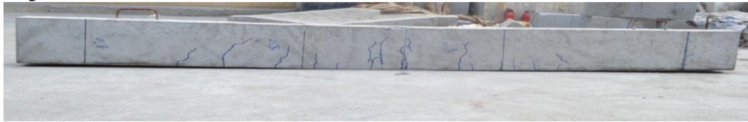
Figure Crack pattern on the specimen
